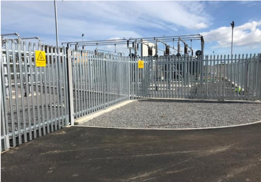
Typical DNO substation complex fencing
