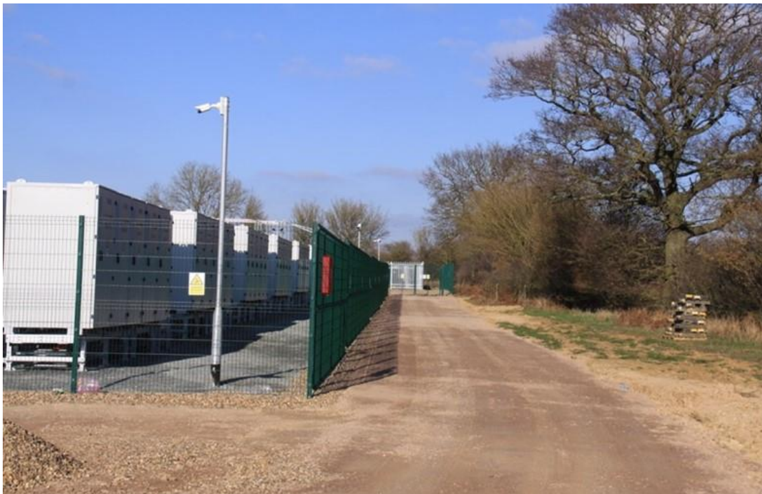
LLPS 17 fencing at BESS site
