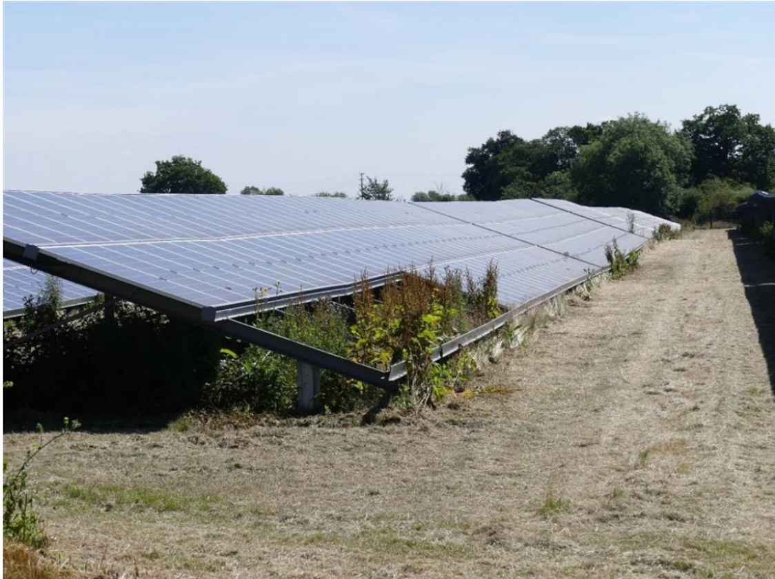
Weeds, left unmanaged, could become a problem for the panels
